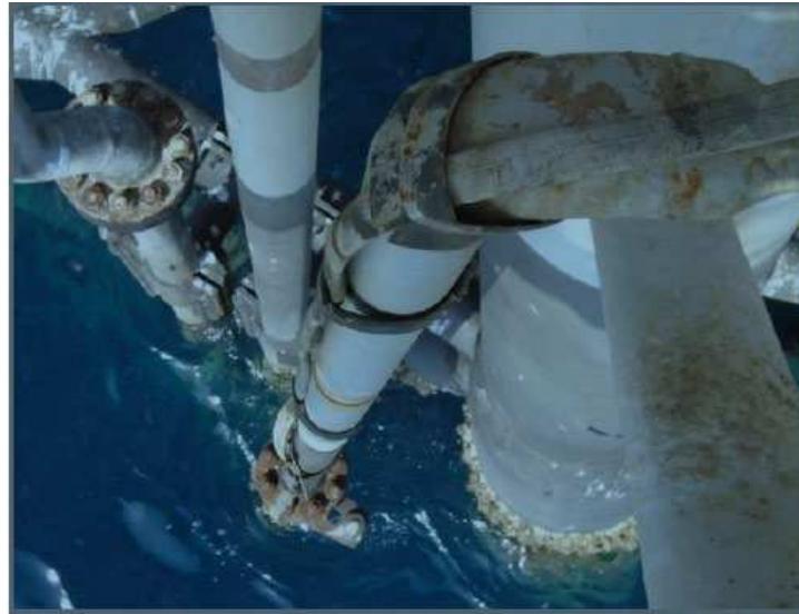
Figure 12. Example of a cable flatpack strapped to a riser.
