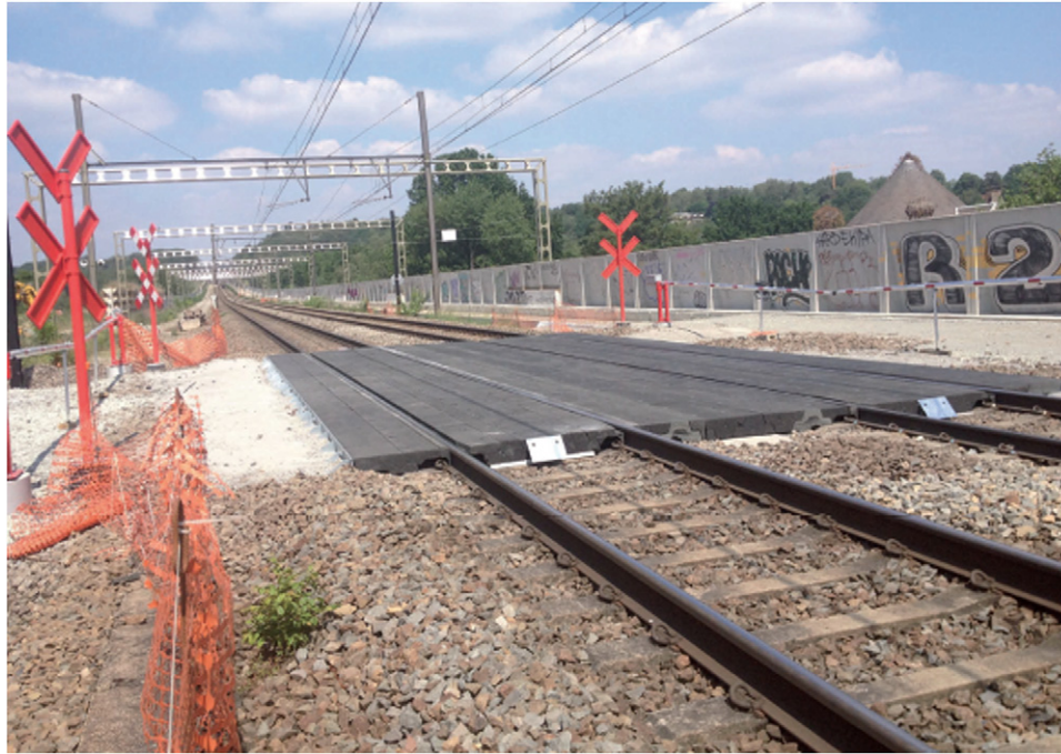
Fig. 17 Level crossing panels including recycled glass reinforced polymer and phenolic from car parts. Courtesy: Reprocover.
